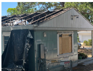
Roof need repair?
